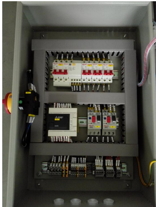
The PLC control panel (5 valve-set up)
