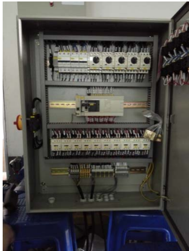
The PLC control panel (5 valve-set up)
