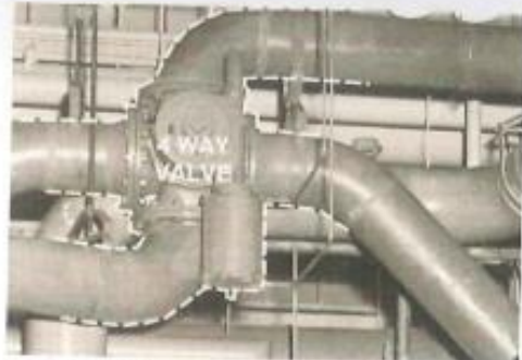
AUTOMATIC VALVE in condenser piping system cycles brushes every eight hours. Flow reversal is followed one minute later by a second reversal which returns flow to forward direction.
